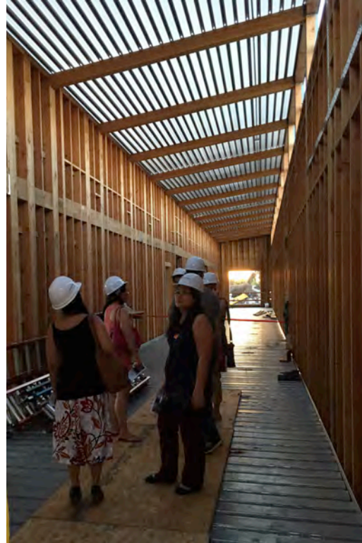
Citizens' Bond Oversight Committee members enjoy the early evening light filtering in through the windows of the second floor of a new two-story building currently under construction at American High School
